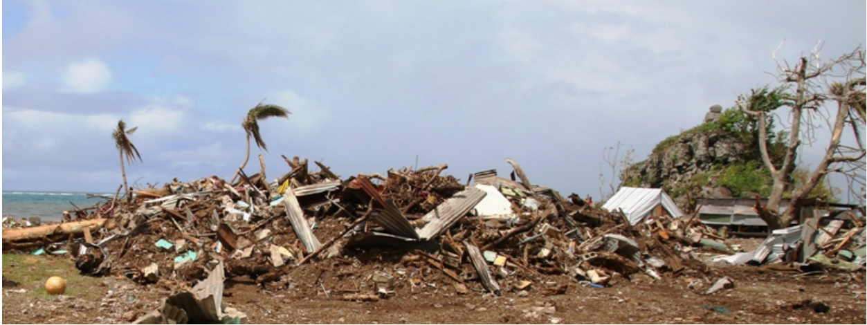
Pic.2 Debris being piled next to the sea
